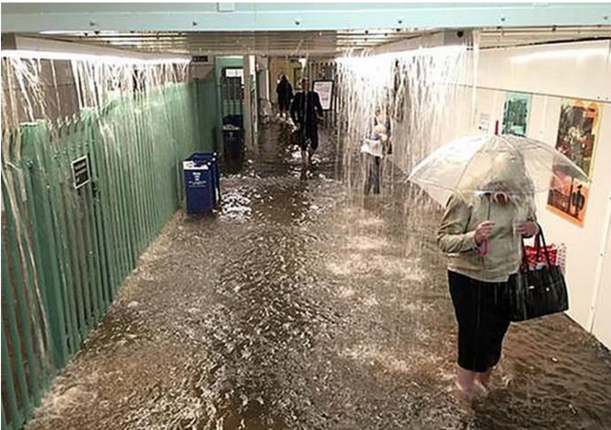
Flooding in Hove station underpass
